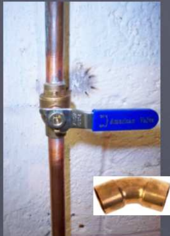
Copper pipes are widely used in central heating systems
